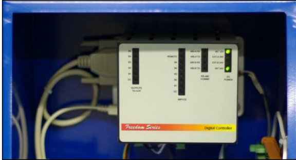
Fig. 3 DCMU adds L-827 Monitoring and IRMS capability to existing CCRs and a redundant RS485 Modbus communications interface to a new 3rd party ALCMS.
