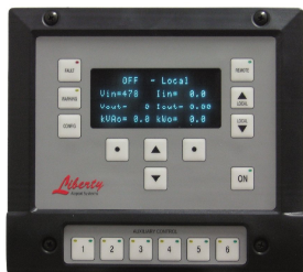
Fig. 1 DCMU Digital Display with auxiliary keypad for control of L-847 Circuit Selector Switches.
