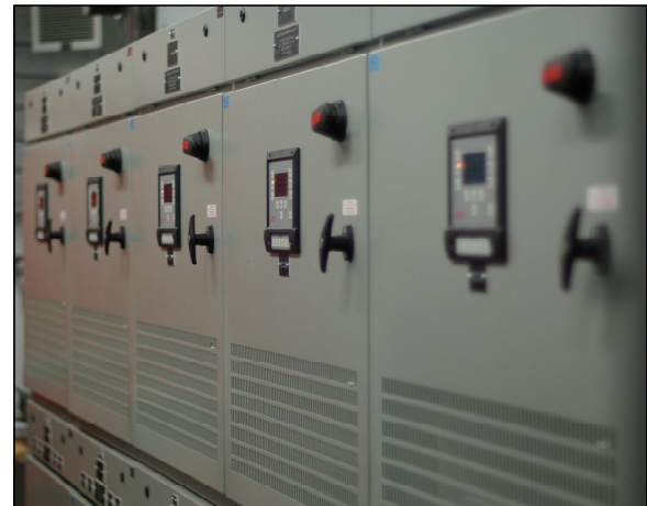
Fig. 3 Freedom Series Switchgear Regulators provide constant current to the airfield lighting circuits.
