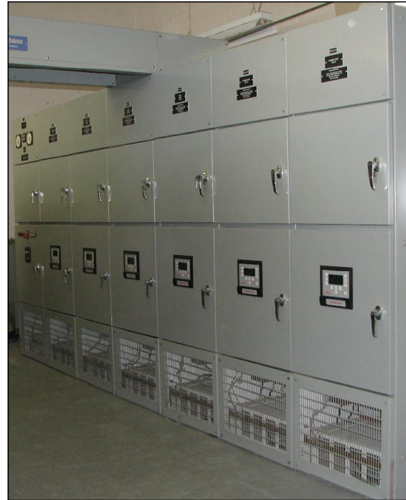
Fig. 2 2400V Liberty Digital Switchgear regulators installed next to existing RSS20 CCR. Cell dimensions are 24"w x 80"h x 31.5"d.
