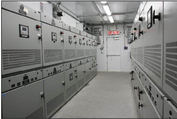
Fig. 1 Two 600V Switchgear Line-ups installed in an Airfield Lighting Field Electrical Center (ALFEC).
