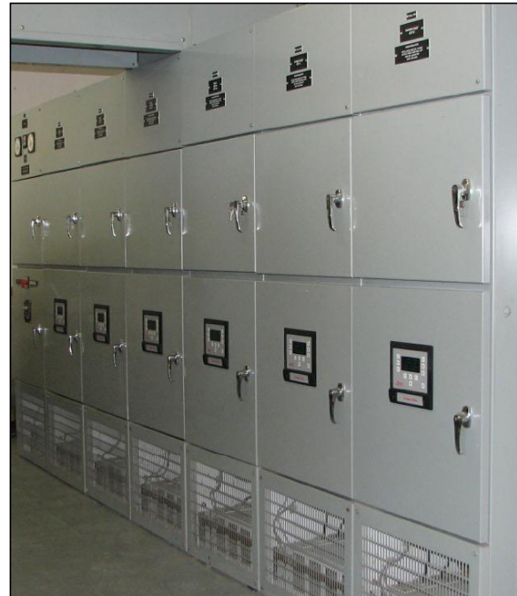
Fig. 1 Liberty 2400V CCRs installed next to RSS20 CCR.
