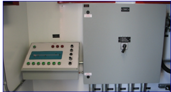
Fig. 4 L-821 Panel mounted in vault next to interface panel.
