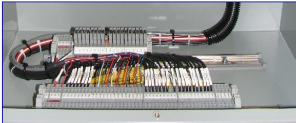
Fig. 2 Terminal blocks provide convenient connection points for customer's wiring to electrical vault equipment.
