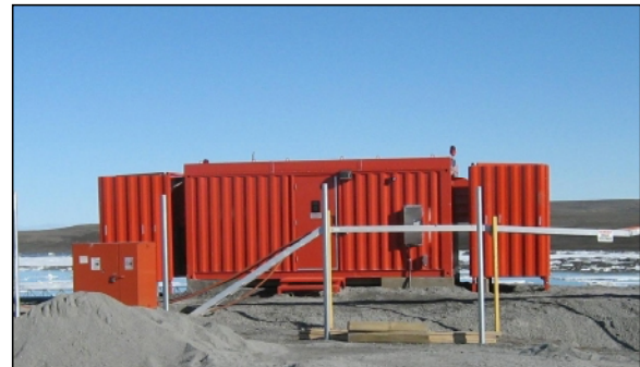
Fig. 1 8' x 20' ALFEC and external wind walls during installation in the high Arctic, c/w 10 Switchgear Cells (Regulators, Circuit Selectors, Non-Regulated Cells), and FM-200 Fire Suppression System.
