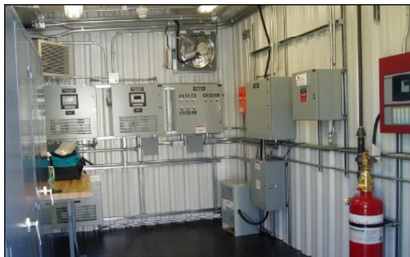
Fig. 2 Spirit Series wall mounted CCRs, Non-regulated panel, ARCAL, ALCMS & Novec-1230 Fire Suppression.
